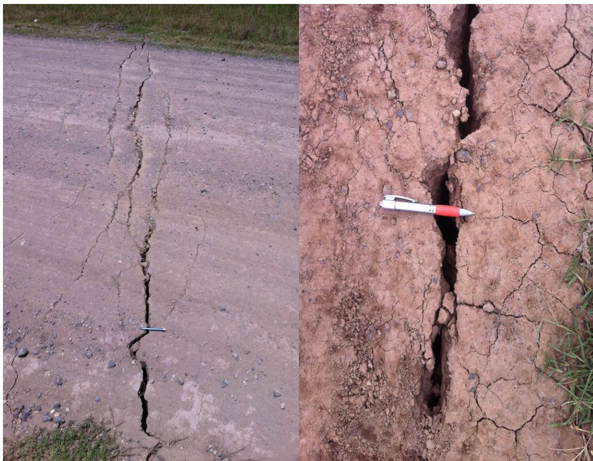
Figure 7: LW7B cracking across the Macquarie Generation access road pre-remediation (28/11/12)
