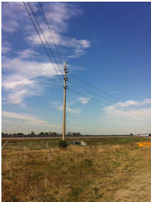
Figure 5: Concrete 33kV power pole (PP35) post subsidence (18/9/12).
