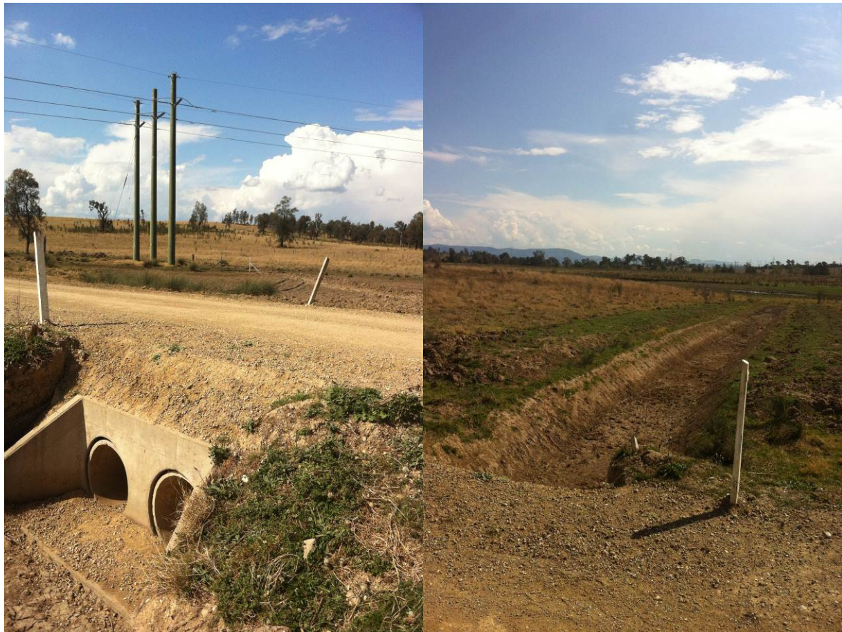
Figure 11: A repair to the culvert under the alternate access road adjacent to 132kV pole set 9 has been completed (over LW6). Water was accumulating around the pole footings and the ground profile was no longer allowing water to travel under the road towards Dam 11.
