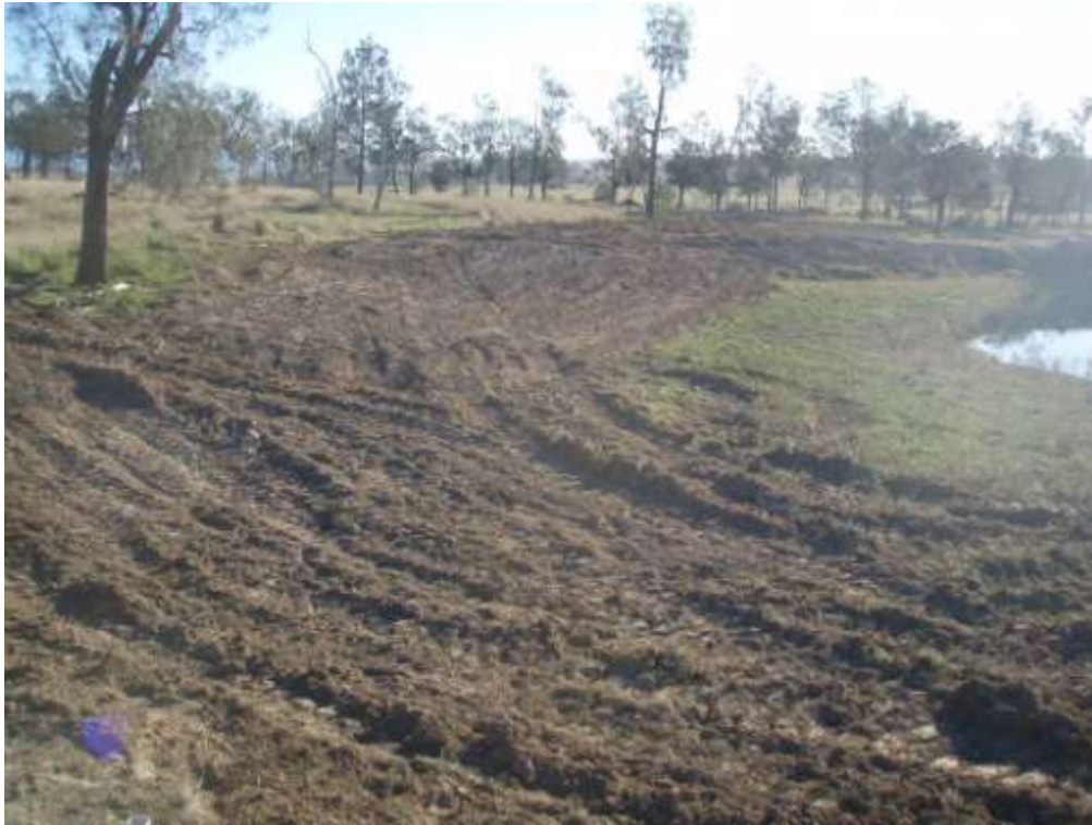
Figure 7: LW4 start line crack (Ref: Figure 6 ) remediated on 25/06/10. Dam re-filling after being drained prior to Longwall extraction.
