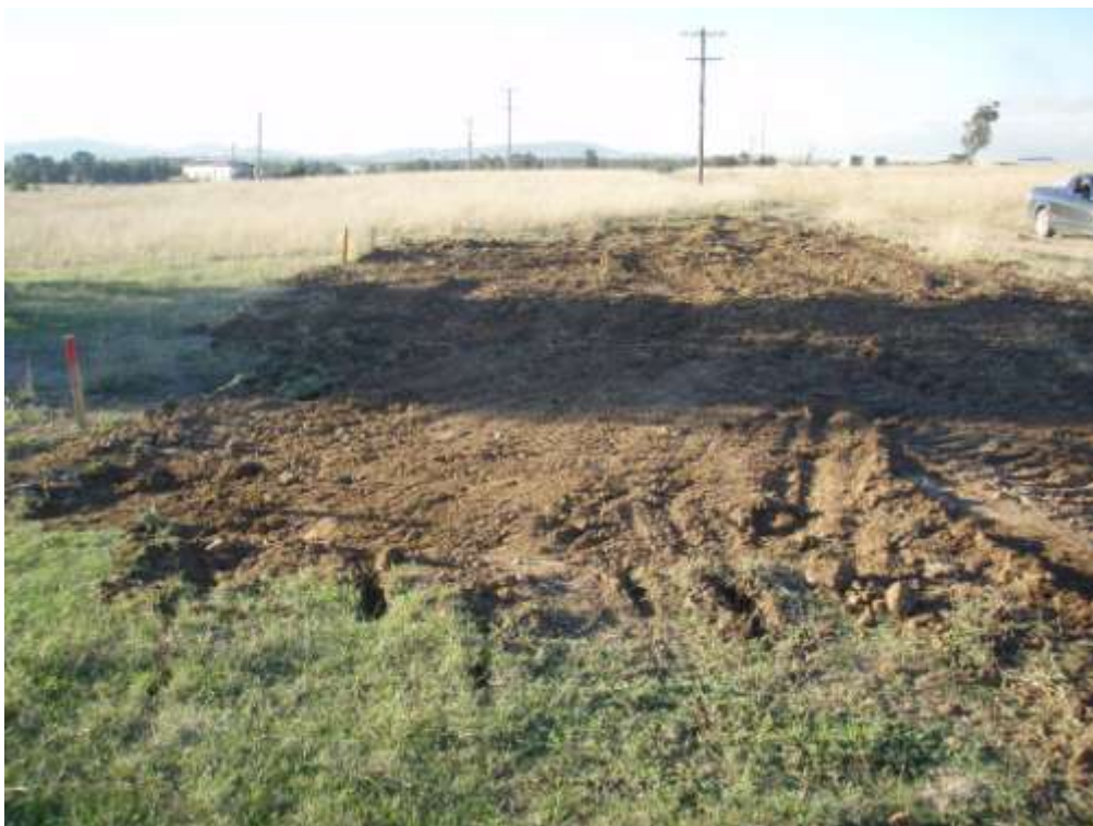
Figure 5: Subsidence Remediation of hole in front of Blue House (Ref: Figure 4 ) looking north from 23/06/10.
