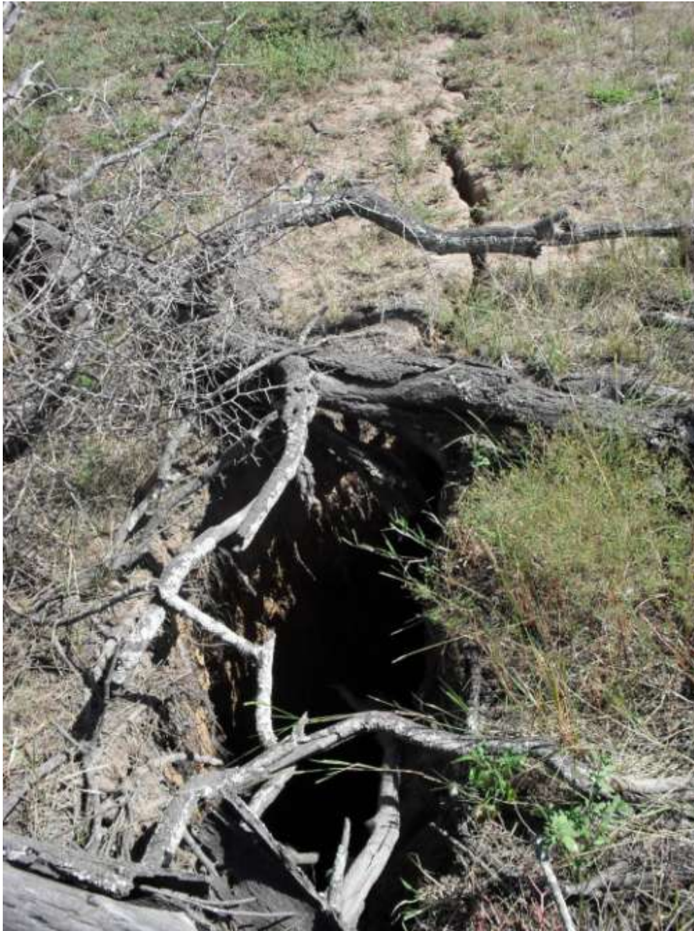
Figure 6: LW4 start line crack in drained dam looking to the west. This crack has formed under a tree located in the southern side of the dam wall.
