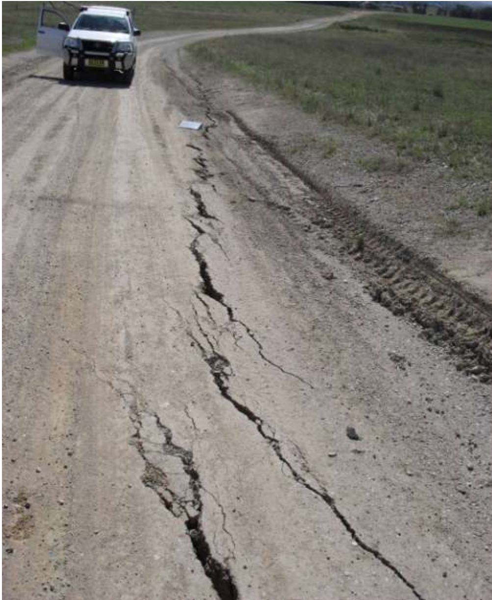
Figure 8: Gateroad cracks in the access road looking north. Remediation required.
