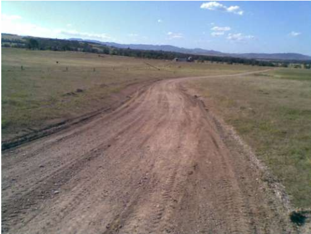
Figure 9: Access road looking north post remediation using a grader with ripping tines on 11/06/10.
