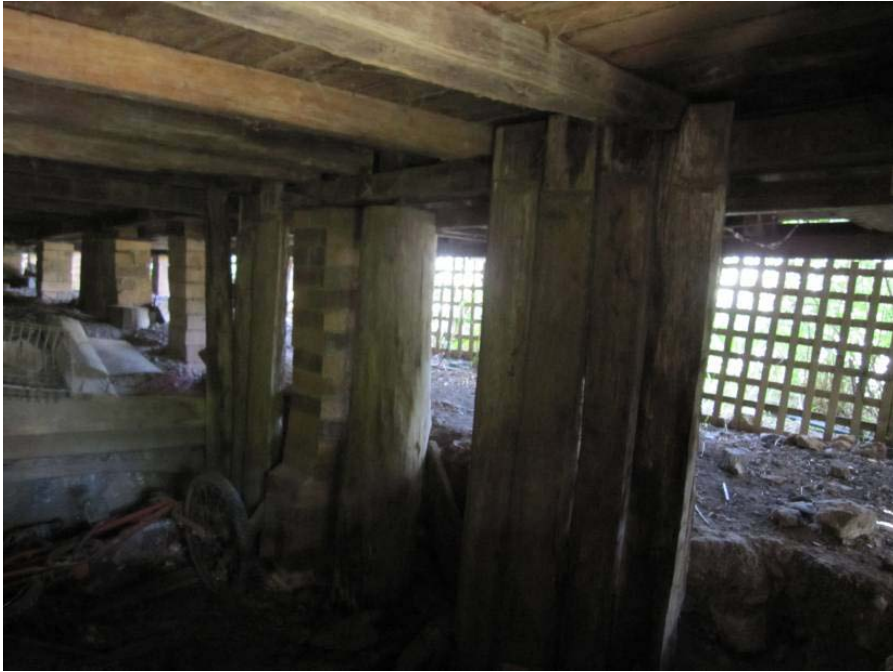
Plate KA-19: Cellar space under original post office room - note new brick piers
