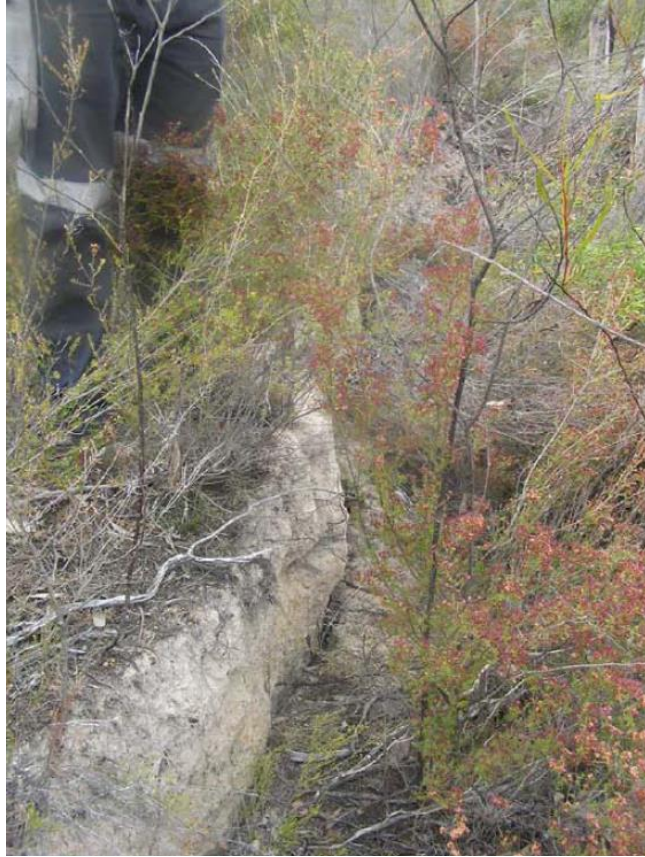
Fig. 4.9 Isolated Surface Step 0.8m high, above Longwall E at Ulan Coal Mine, 260m void width, 1.31m maximum observed subsidence, 130 to 145m cover. (Ulan Longwall E End of Panel Subsidence Report)
