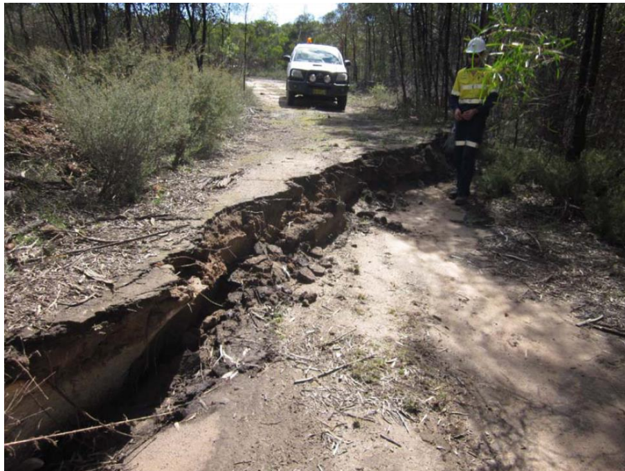
Fig. 4.8 Surface Step 0.5m high, above Longwall C at Ulan Coal Mine. 260m void width, 1.27m maximum observed subsidence, approximately 180m cover. (Ulan Longwall C End of Panel Subsidence Report)
