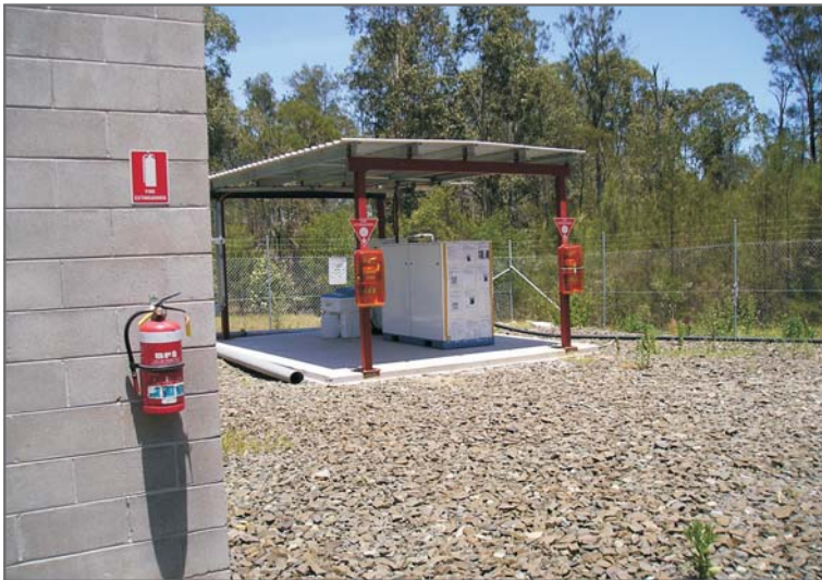
Photograph 4 Existing nitrogen inertisation plant.
