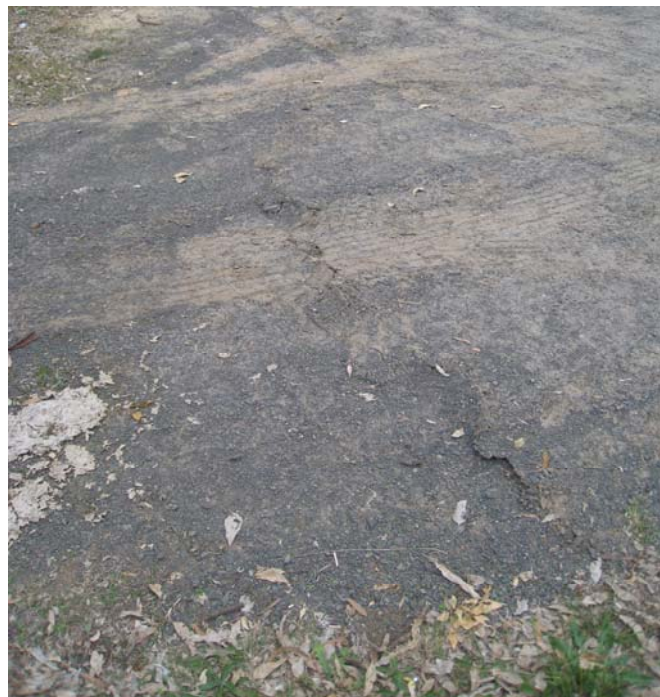
Fig. 4.6 Example of surface compression buckling observed in road pavement (observed in the southern coalfield at a similar depth of cover as the Study Area)
