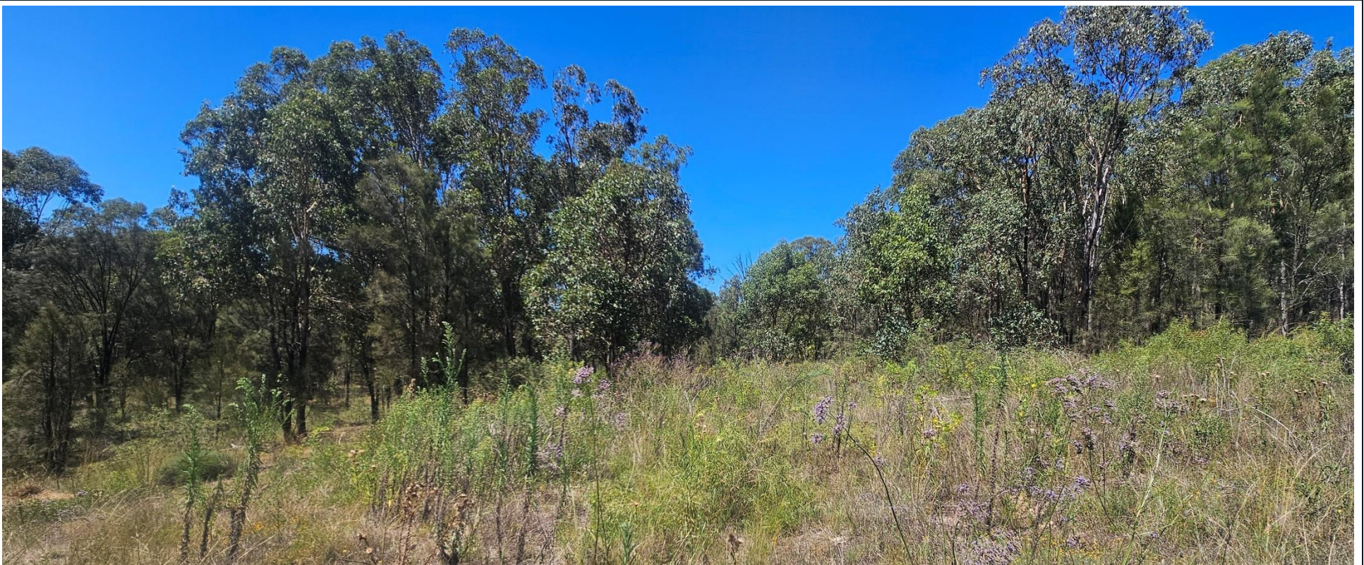
Plate 14 SWCA – Remediated subsidence cracking within Underground Woodland Monitoring Site (SVCA05), facing south
