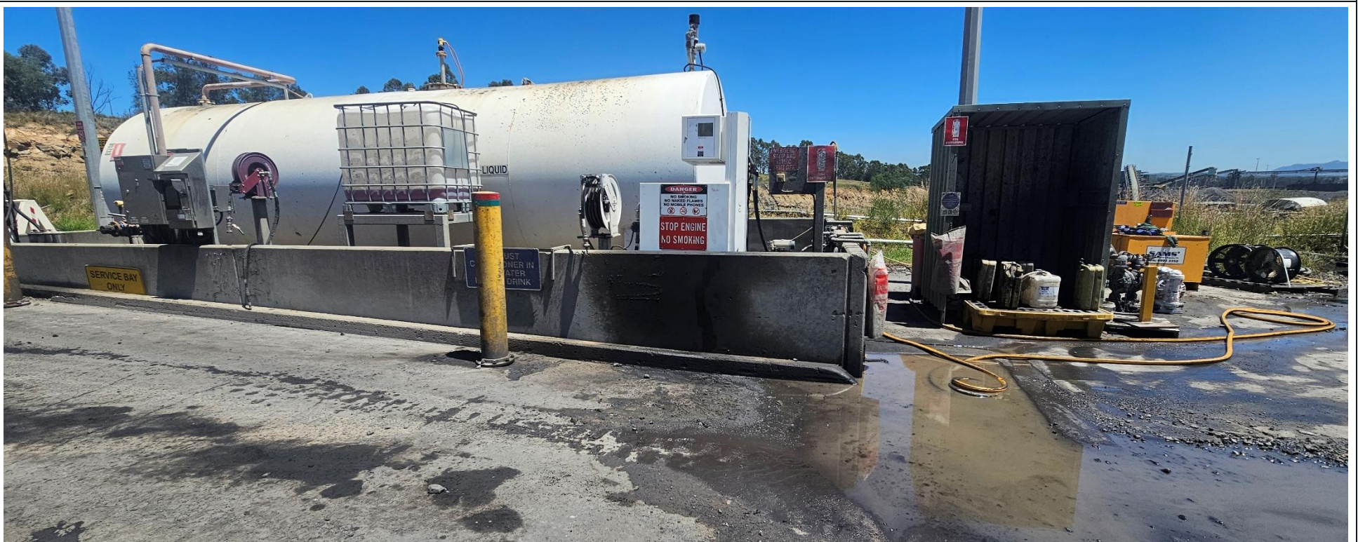
Plate 23 Bunded diesel storage at the Mine workshop
